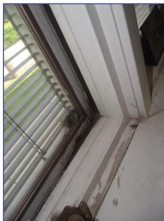
Figure 8: Window with Frame Damage
