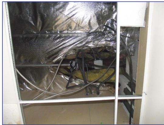
Figure 7: Ceiling Leak in Lobby of Police Area
